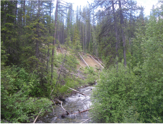
Photo G – Natural, existing bank failure upstream of the second crossing of the Mark Creek mainstem (GPS 095). Note the green-up along the toe.
